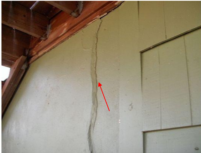
Rear masonry foundation wall cracked displaced and no longer plumb
