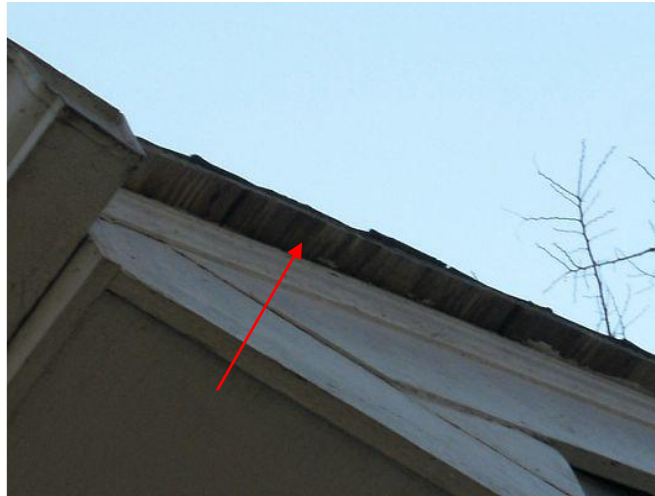
Exposed plywood roof decking
