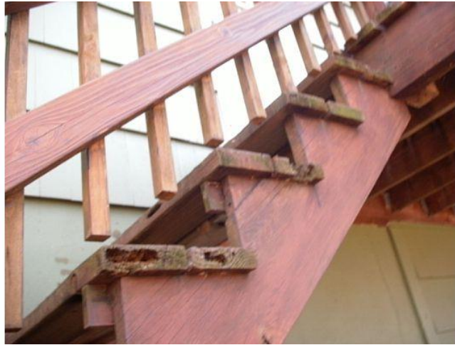
Deteriorated stair edges
