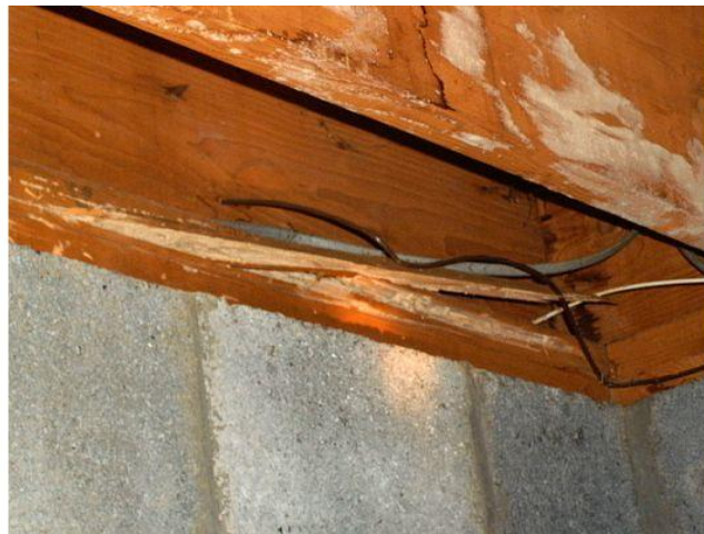
Termite damage to the sill plate
