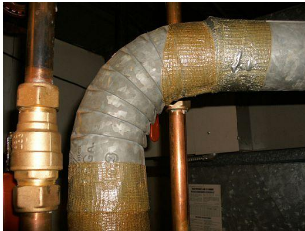
Old hot water flue pipe improperly installed
