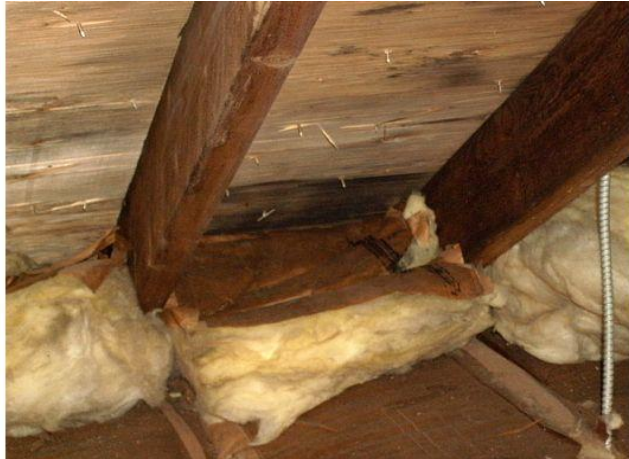
Stained area of roof sheathing due to moisture condensation or leaks
