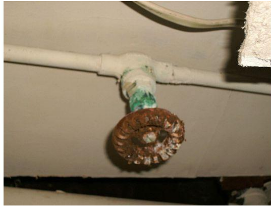
Corroded shutoff valve suggests leakage
