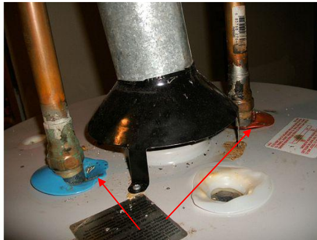
Melted trim rings indicate problem or hazard
