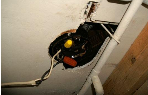
Open junction box and loose cable above drop ceiling are a hazard
