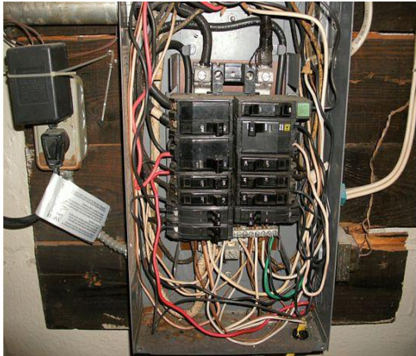
Obsolete breaker panel without single main breaker
