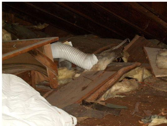
Bathroom vent fan discharges into attic
