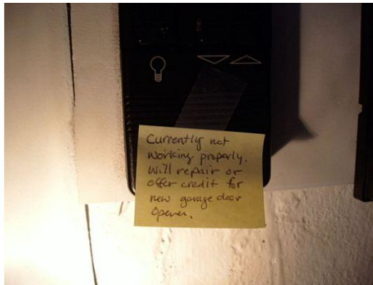
Note on opener indicating it does not work (placed by seller)
