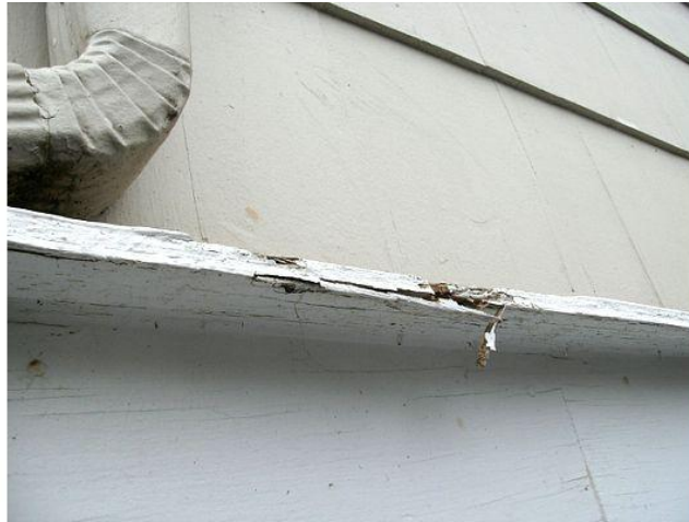
Water damaged exterior wood trim
