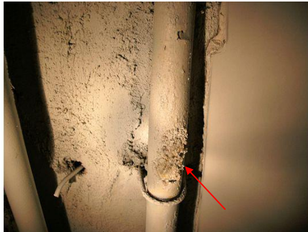
Leaking brass water pipe found in garage
