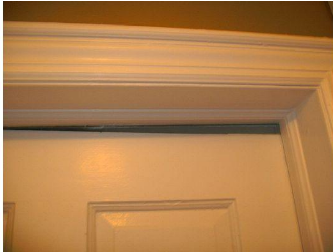
Gap at top of door
