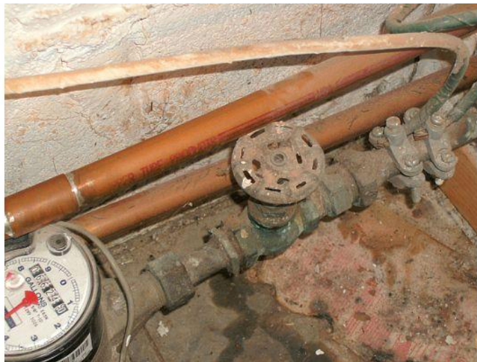
Older shutoff valve
