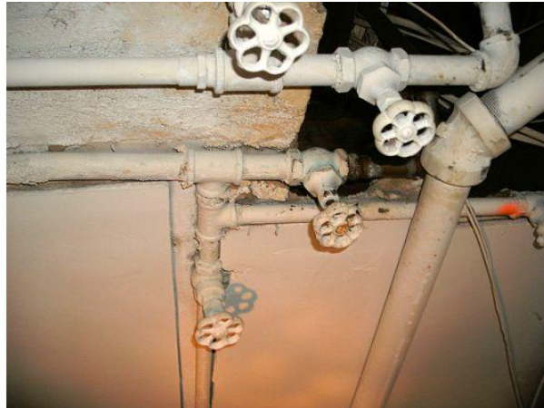
Old brass water pipe
