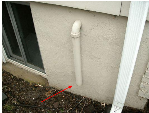
Sump pump discharge pipe discharges at the base of the home
