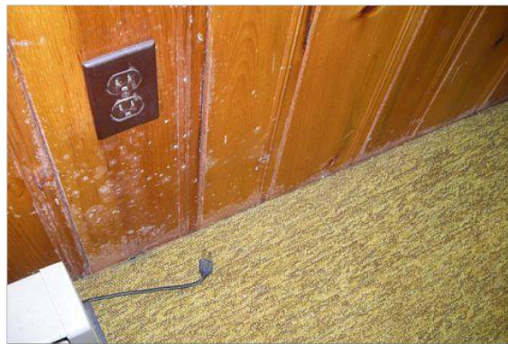
Spotting from mold growth on wood panels
