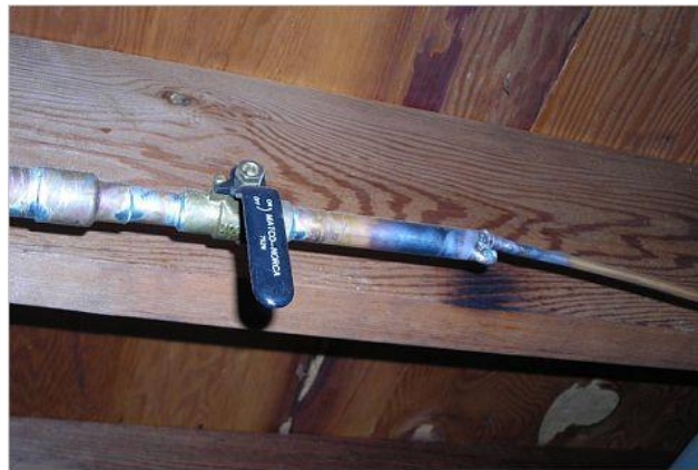
Poorly done connection
