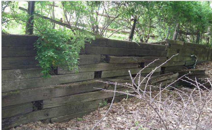
Wood rear retaining wall has failed
