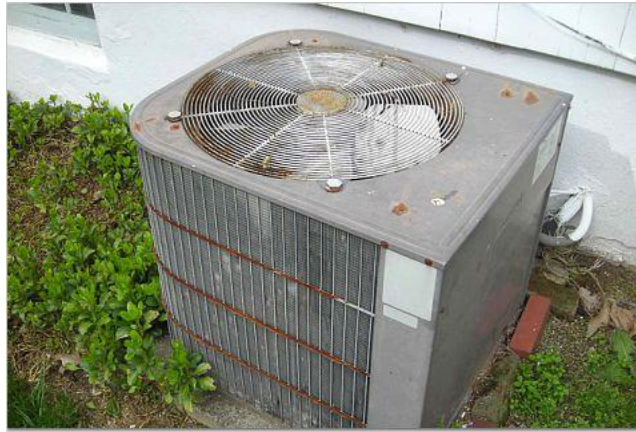
Aging AC equipment with corrosion
