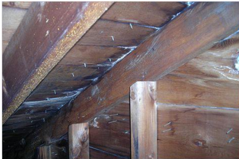
Stained areas in attic indicate roof leakage
