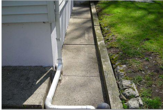
Path section lower than tie wall
