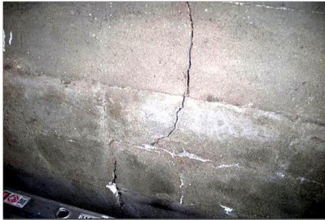
Crack in garage wall, on right side
