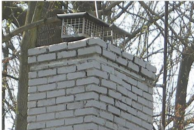
The chimney brick is painted white, but joints still requires re-pointing
