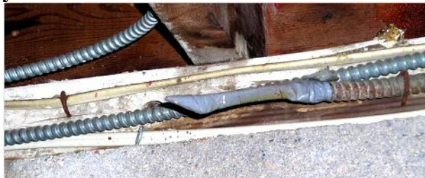
Taped off unused cable in basement
