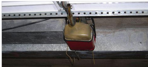
Older openers have no sensors, and are plugged in with extension cords
