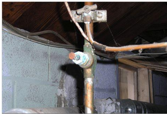
Old shutoff valve with missing knob
