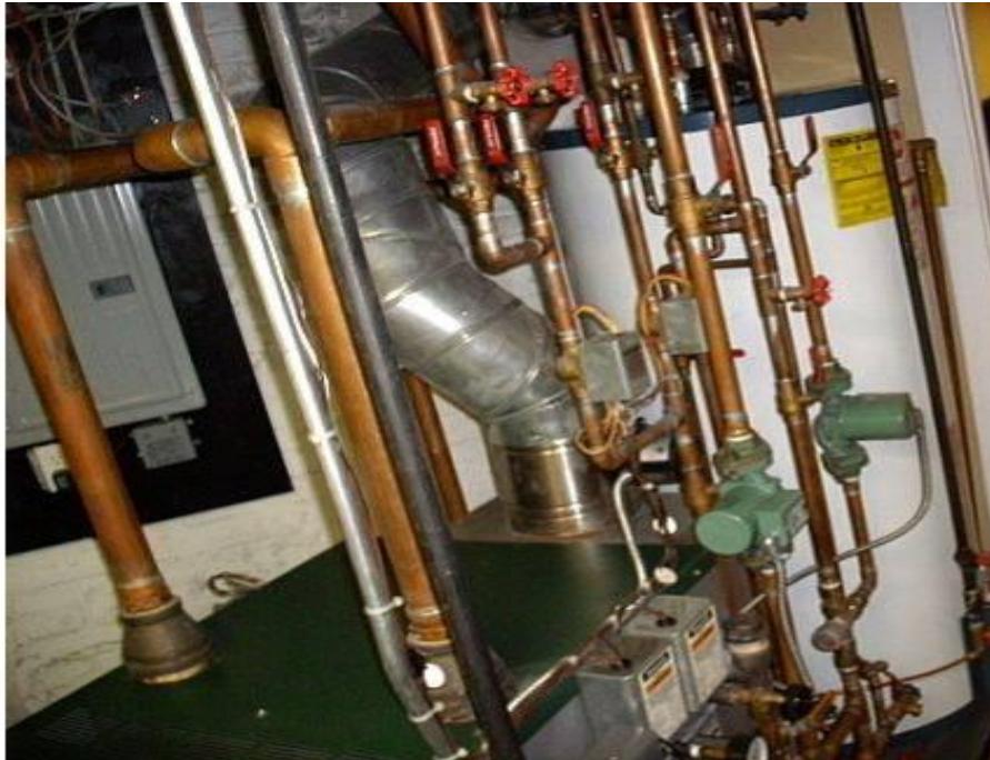
Heating System is Combination of Steam and Circulated Hot Water from Same Boiler
