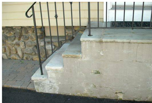
Masonry Steps at Side are in Only Fair Condition
