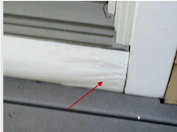
Deteriorating threshold board
