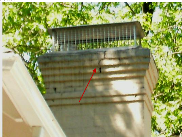
Cracks in the masonry chimney visible at top
