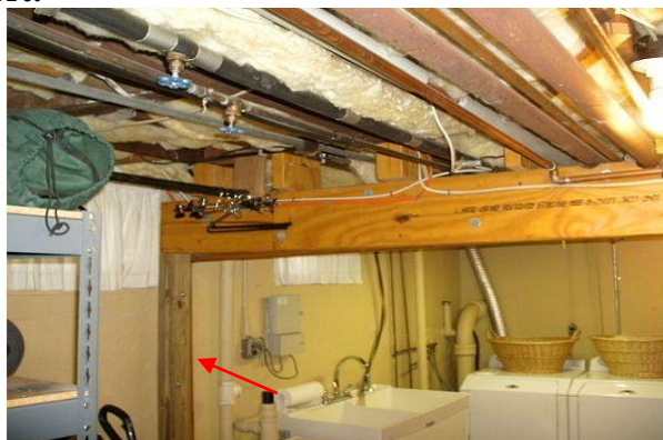
This Wood Post Support May Not be Adequate
