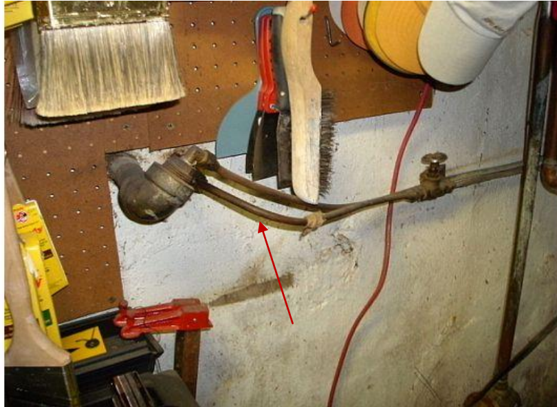
Old fuel oil lines passing through wall suggest that a buried tank may be present
