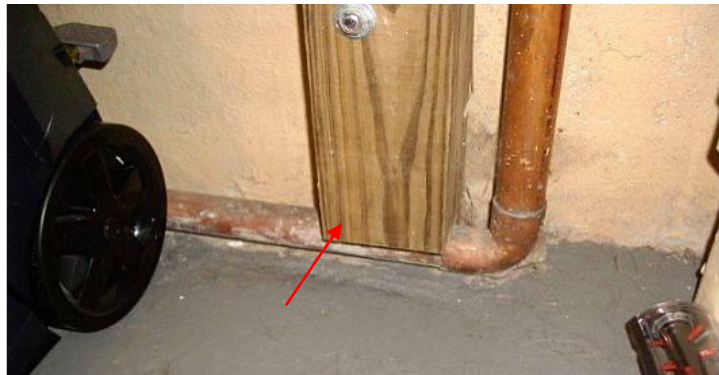
Support post notched over heating return pipe and not on footing
