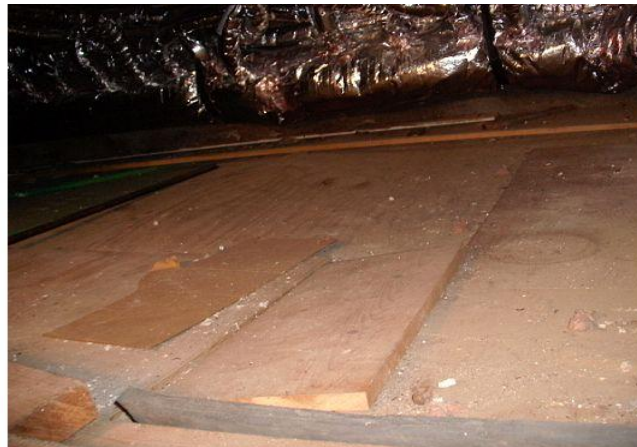
Wood in contact with soil on the crawlspace floor
