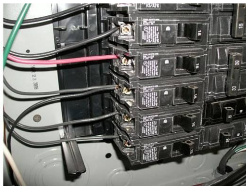
Double tapped breaker in sub panel
