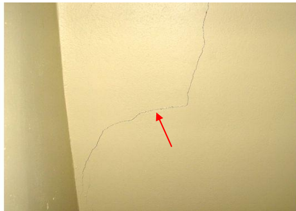
Plaster Wall cracked near chimney
