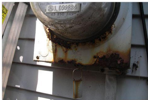
Rusty meter housing
