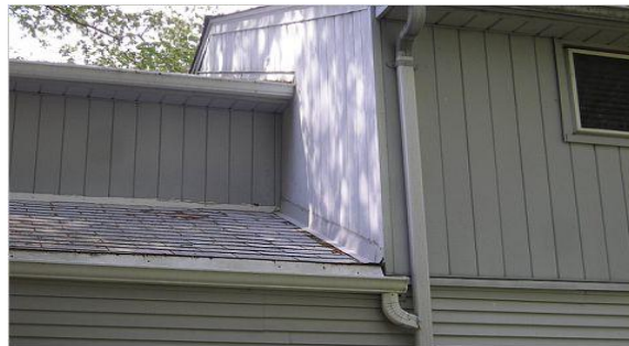
All three major rear roof areas and gutters ultimately feed one downspout
