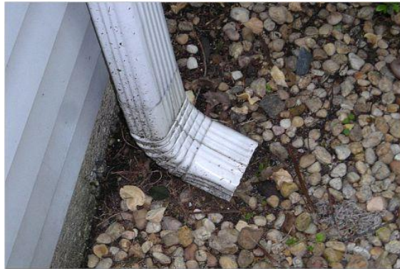
Downspout discharging at base of home
