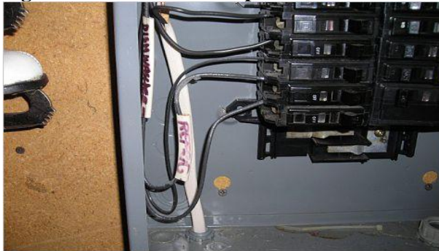
Long white cable – excess insulation in the panel
