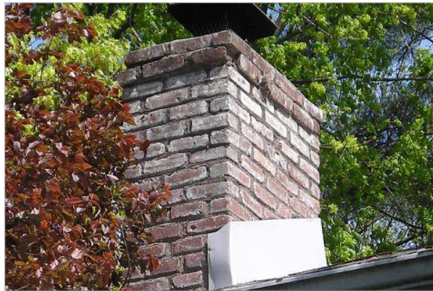
Brick joints appears to be soft and flashing not installed properly
