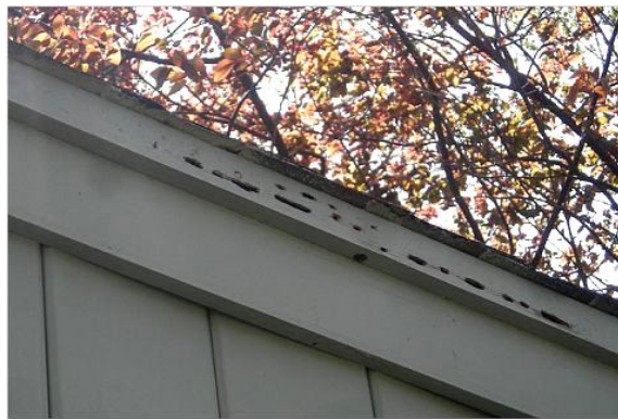
Carpenter bee damage to wood trim
